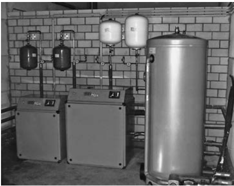
Figure 17.5 Two heat pumps installed according to customer's wishes: on the left, heat pump for heating the left side of the hall, and on the right for heating the right half of the hall and offices
