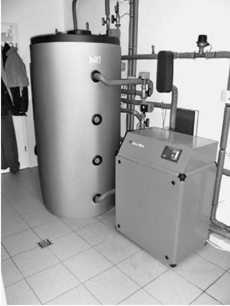
Figure 17.3 Example of a water-water heat pump system with hot water tank and buffer tank, GeoMax® model
