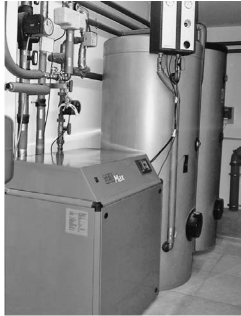
Figure 17.4 Example of a brine-water heat pump with low-flow solar system for hot water generation, GeoMax® model
