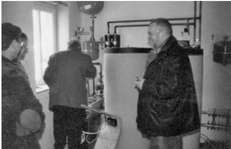
Figure 17.7 Example of a brine-water heat pump system with hot water tank and buffer tank during start-up in a detached house
