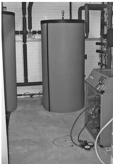
Figure 17.1 Example of a brine-water heat pump with hot water tank and buffer tank, GeoMax® model being put into operation
