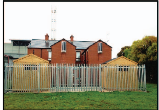
Fig. 3 Platform and sheds for heat pump-storage set-up
