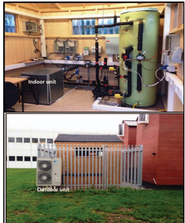
Fig. 4 Heat pump indoor & outdoor unit along with storage tank
