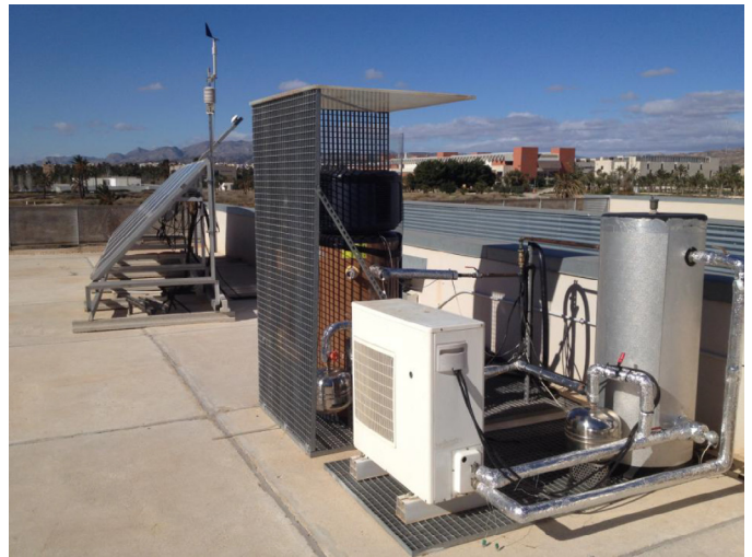
Fig. 1. Photography of the experimental facility.
